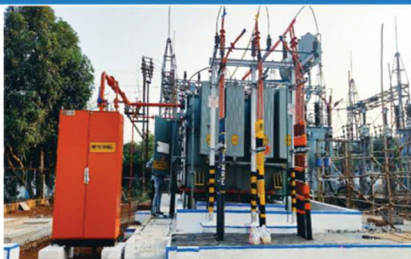
Upgradation of PTR at Sainik School
