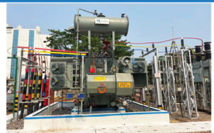
Upgradation of PTR at Kalinganagar
