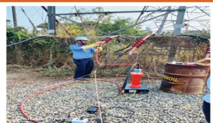
PD of cables to identify weak joints
